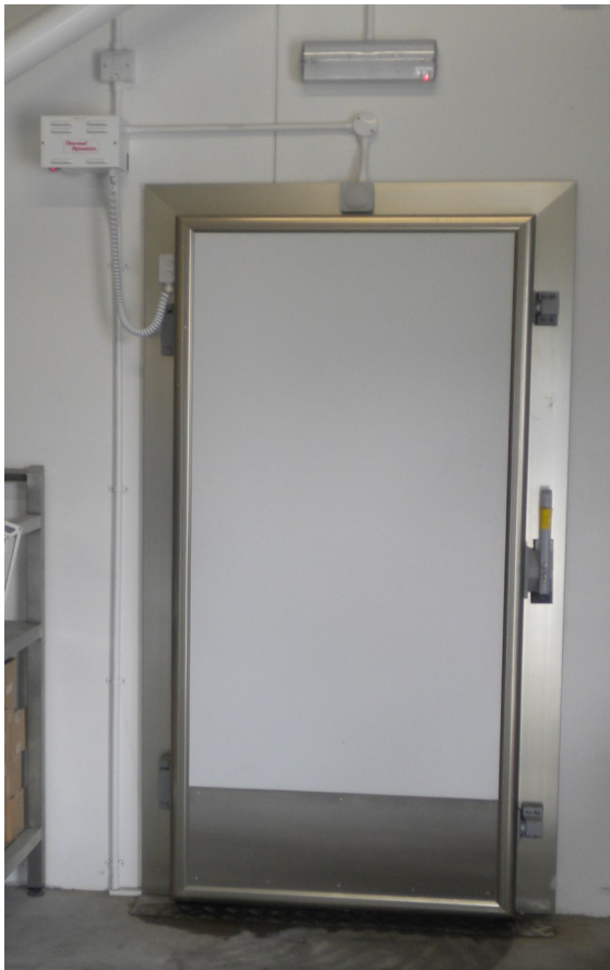
Low Voltage Heater Cable and Transformer for Freezer Doors .
