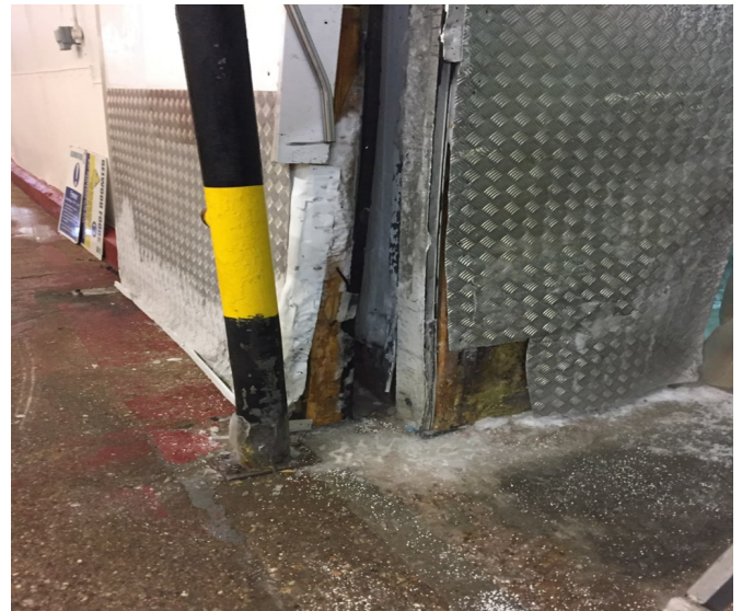
Door damaged by impact
